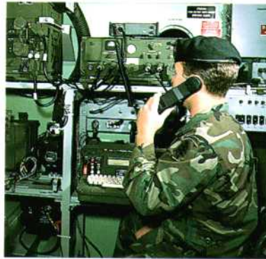
Fixed DSP 9000 base station installation in a communications shelter.
